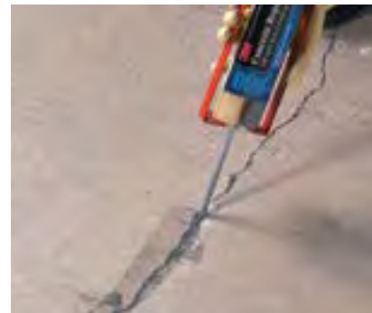
Fix cracks, spalls, and breaks in concrete:
